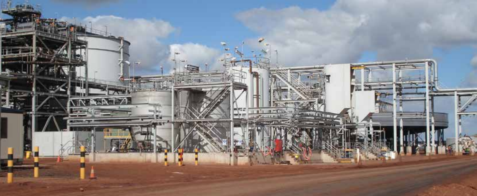
A large scale bespoke flocculent and reagent preparation system installed in a mineral processing plant.
