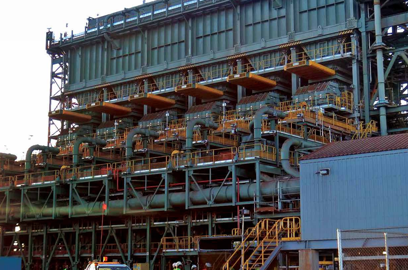
Multiple bin isolation gates on-site in Western Australia.
