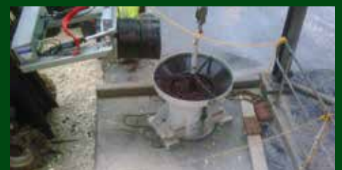
Hoist operated kibble option is the simplest solution for low ball consumption.
