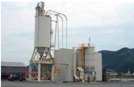
Complete bulk intake and storage facilities.
