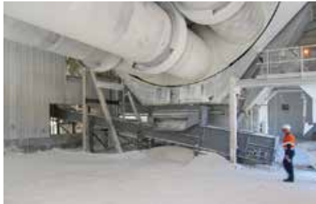
High temperature handling solutions. In this case, quicklime up to 600°C.
