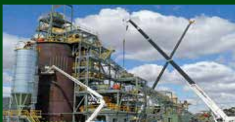
Typical Transmin lime silo during installation at a Western Australian gold mining operation.
