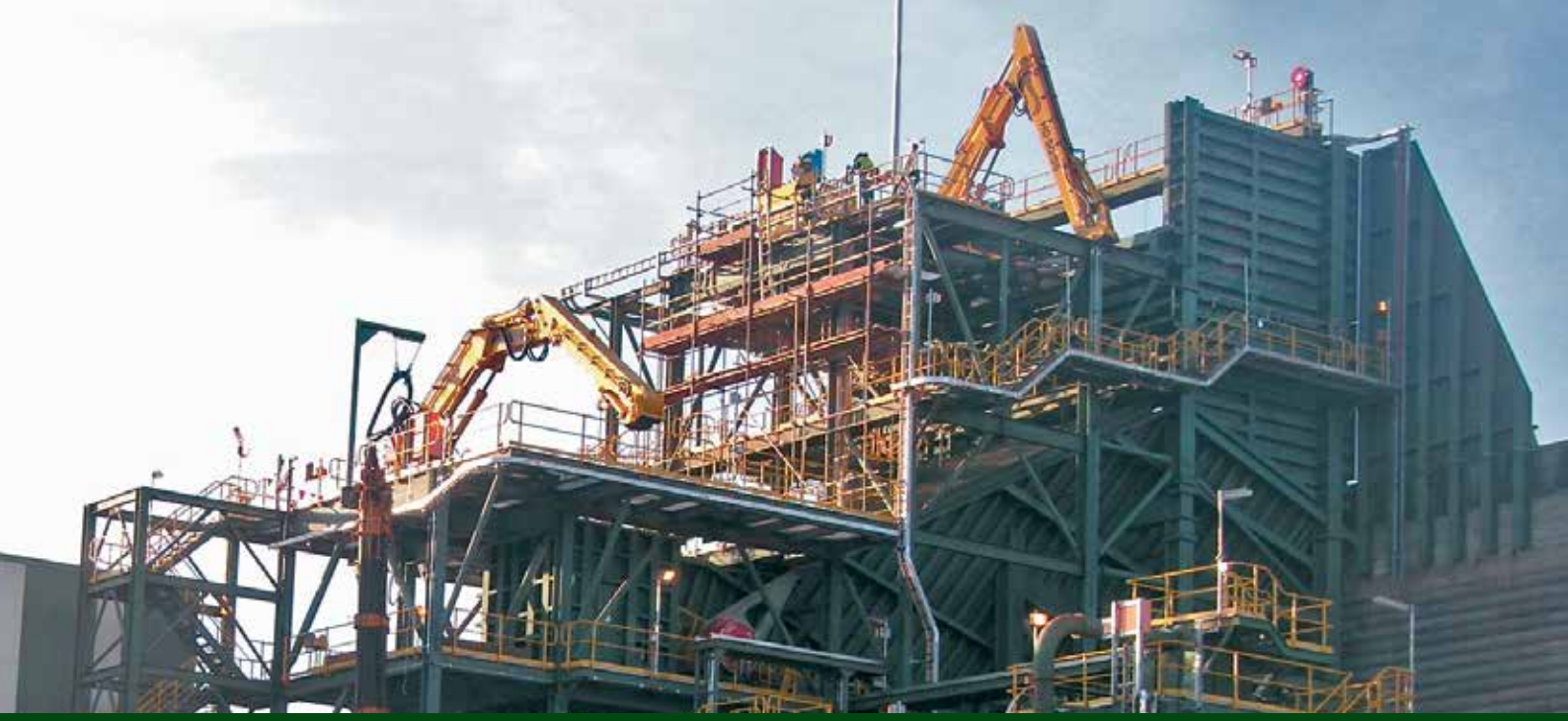
Multiple pedestal mounted rock breakers in the Pilbara.
